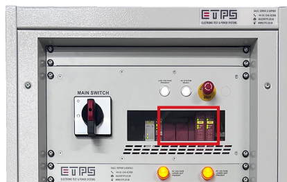
SAFETY RELAY WITHIN MAINS INTERFACE UNIT
